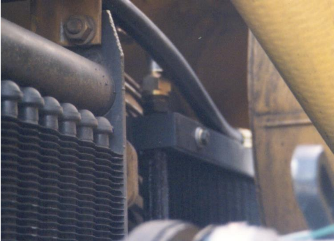
Fittings at top of condenser (view from inboard – right side).
